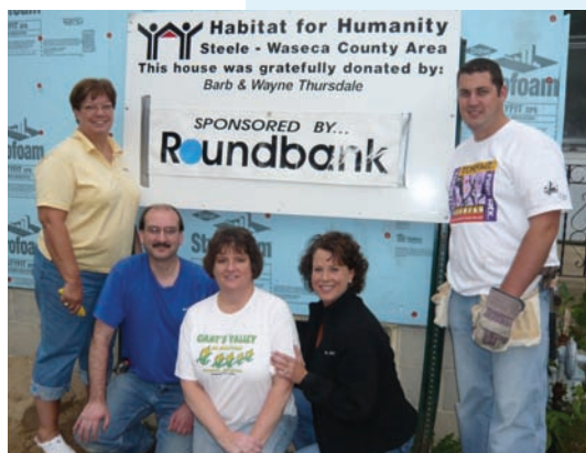
Community members work together to renovate the first home for Habitat for Humanity of the Steele-Waseca Area.
